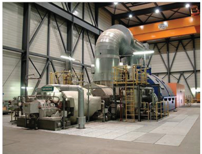
Figure 4 | A steam turbine installation.
